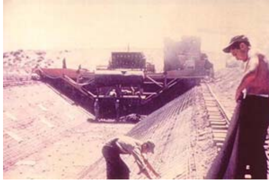
Columbia Basin Canal under construction. Image Courtesy of the Moses Lake, Washington Chamber of Commerce.
